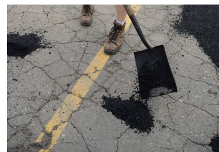
Asphalt Surfaces – Inspections/Repairs
