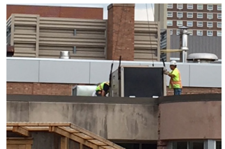
HVAC, Boiler and Electrical Systems Inspections/Repairs
