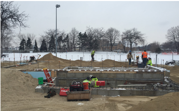
Currie Park Construction began in September on improvements from the park's master plan, including a new splash pad, restroom building and basketball court, in addition to playground safety fencing and path and lighting improvements. A grand opening is planned for summer 2020.
