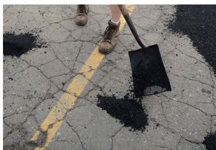
Asphalt Surfaces – Inspections/Repairs
