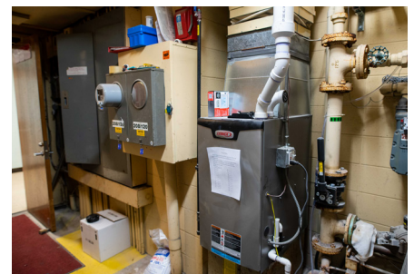
HVAC, Boiler and Electrical Systems Inspections/Repairs
